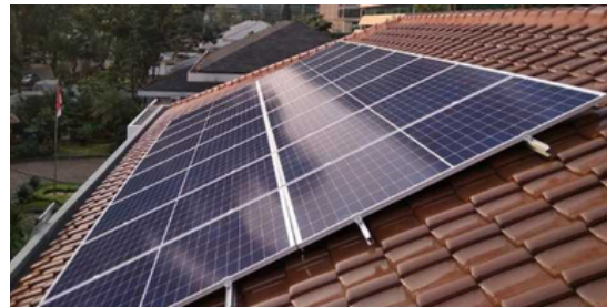
UNY Solar Panel at Rooftop
